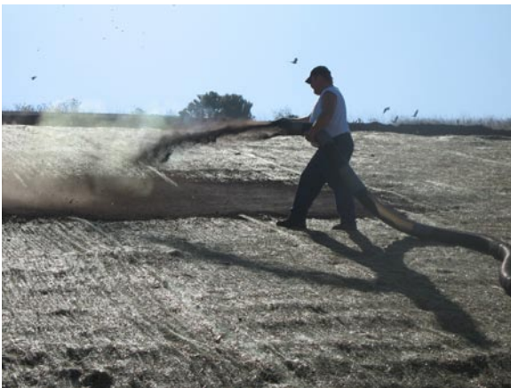
September 24: Compost applied by blower over coconut erosion blanket. Seed was injected into the compost by blower truck.
